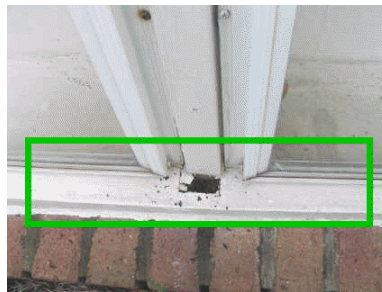
Sill rot behind aluminum
