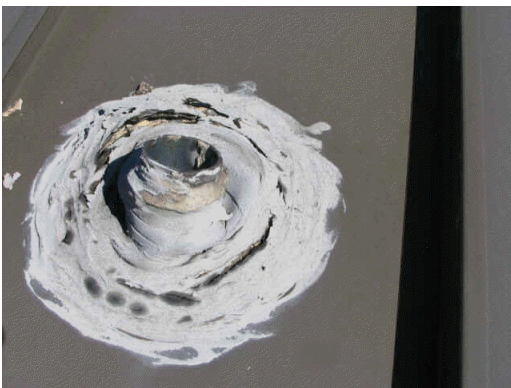
Roof flashing deteriorated on the left side.
