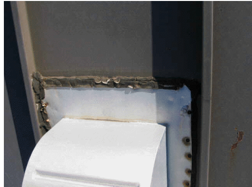
Sealant deteriorated around roof vent.
